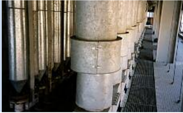
KHARG - Burner Row
