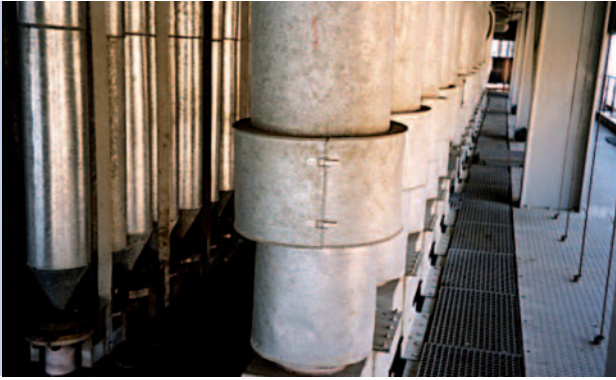
KHARG - Burner Row
