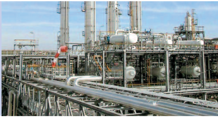
Butadiene Plant, Germany
